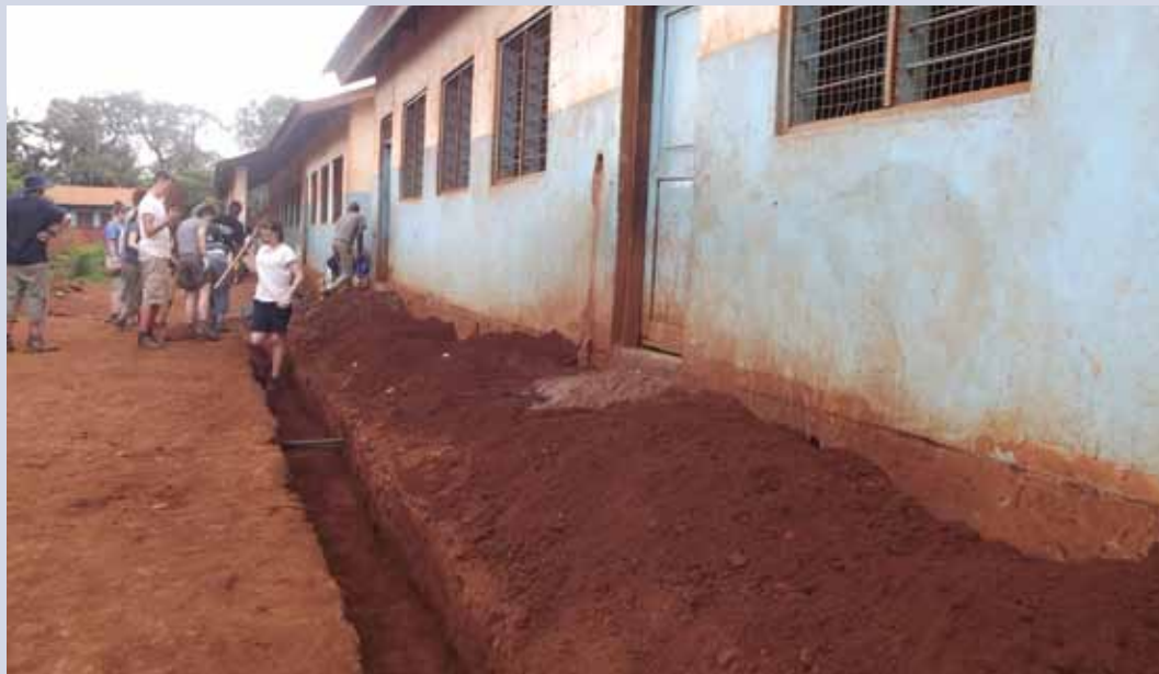
Figure 1. Part of the trip included renovation of buildings in the local village.
